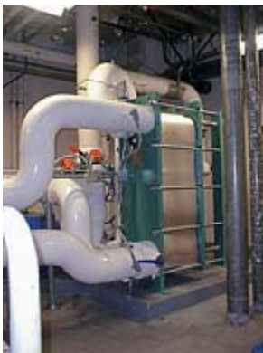
Figure 2. Heat Exchanger Used in Free-Cooling Application
